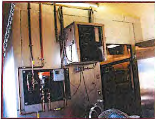
Concrete Moist Room
